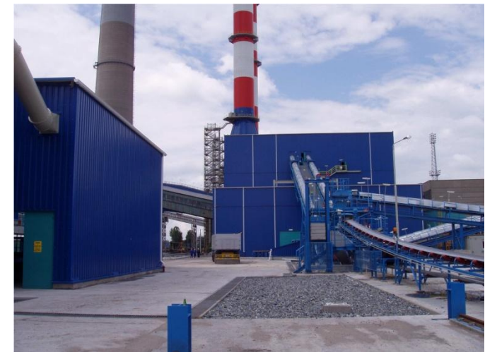
Lime Store Handling for the Flue Gas Desulphurisation Installation at Maritsa Istok III Power Plant
