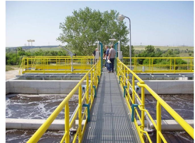
Water Treatment Plant at Maritsa Istok III Power Plant
